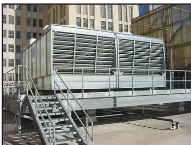
3,000 ton condenser water plant
