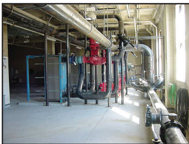
Complete new HVAC systems
