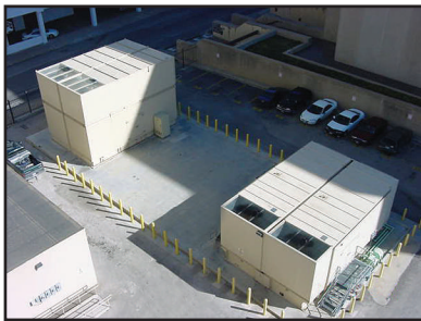
Generator pad with conduit to accept tenant installations
