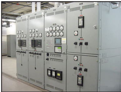
Emergency generator electrical paralleling gear
